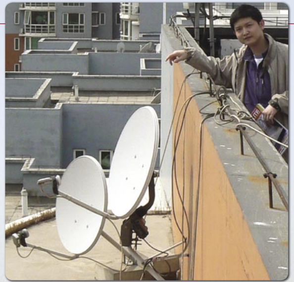
■ Additional antennas are mounted on a side railing: a 75cm dish is pointed to 134°E with a 60cm antenna motorized with a MOTECK motor.
