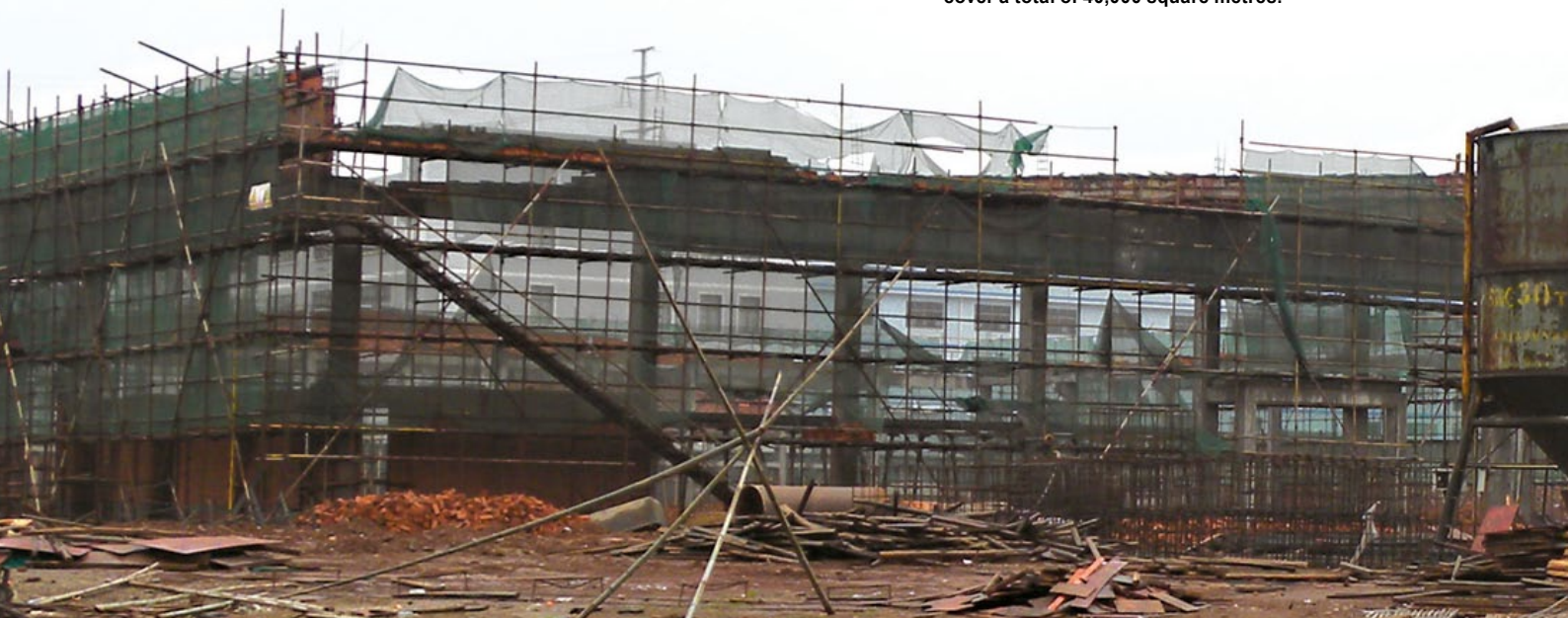
■ Construction site of the new production hall which will cover a total of 40,000 square metres.
