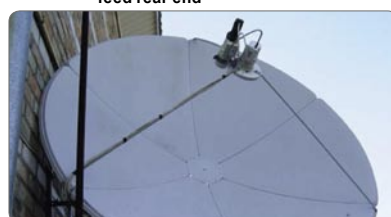
After some finetuning, in less than 2 hours, Sergey could double the amount of channels he received by adding Ku-band to his system.
