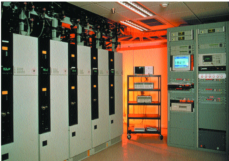
Fully automated klystron power amplifiers
