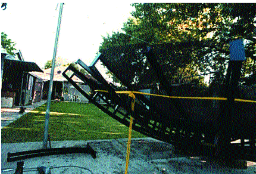
As well as support when the dish is in its early construction phase this rope is gradually tightened and draws the dish up so as the rim can be fitted.
