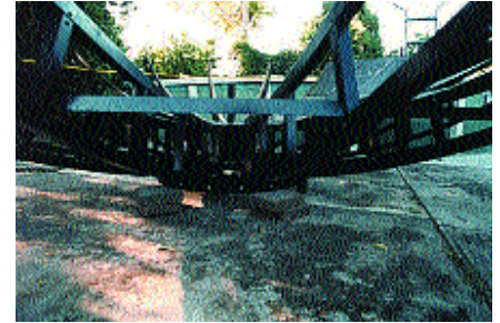
Supports and bracing need to be loosely bolted together to allow flexibility. The mounting ring was sat on three bricks to allow clearance underneath and to tilt the dish for fixing of bolts.
